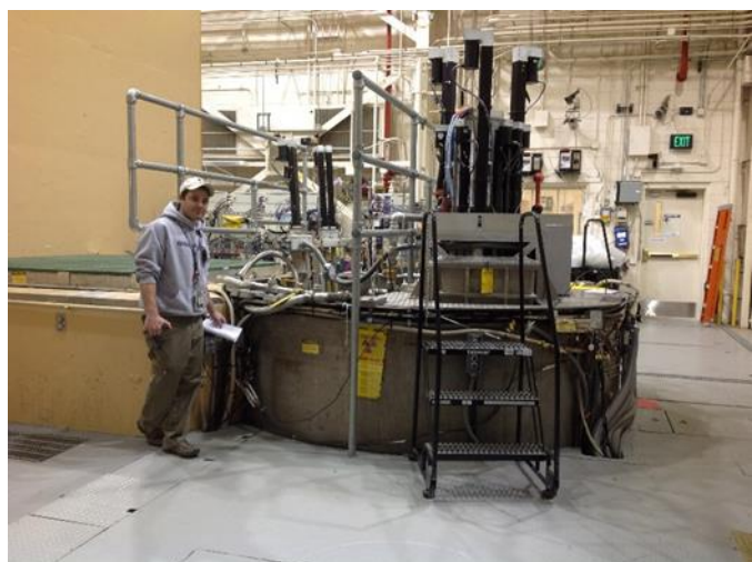
Figure 3 - View of the rod control drive motors (and me) surrounding the opening for the central cavity
